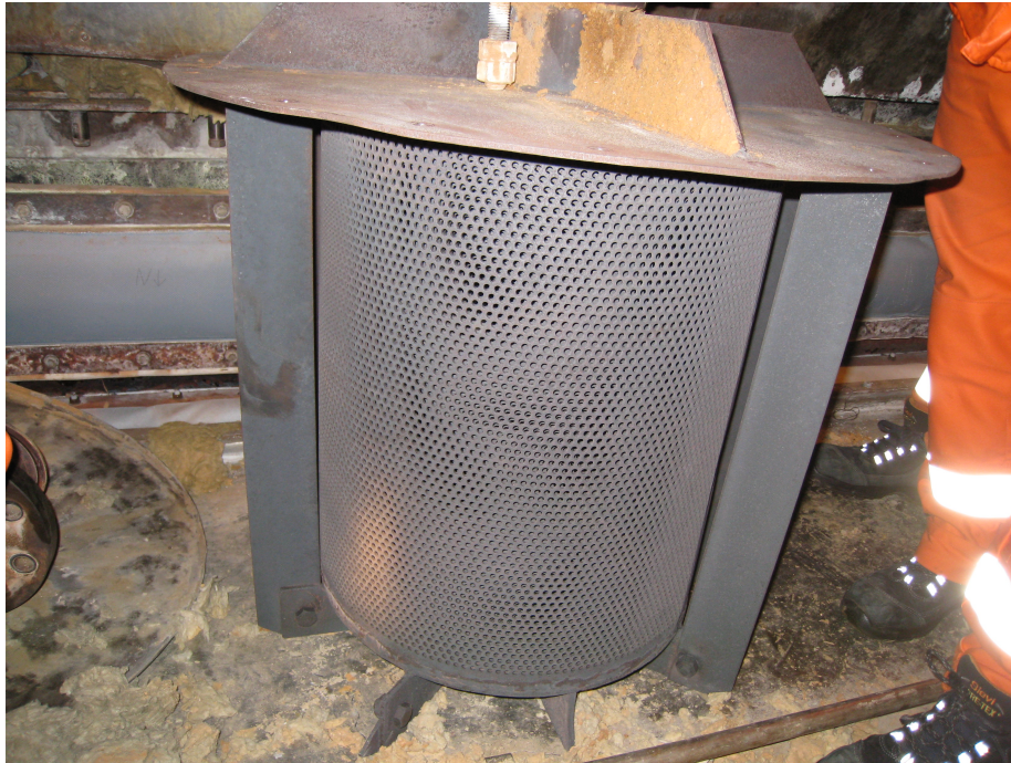
Figure 1.2: Revision A of the diffuser after inspection. It can be seen that two of the supporting rods have detached from the diffuser and are no longer serving their intended purpose. Photo provided by Mjørud AS.
