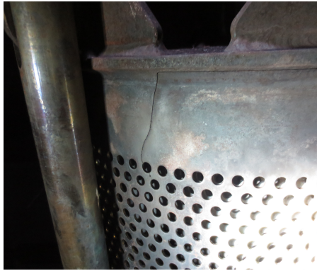
(a) One of the cracks found at the top of the diffusor.
