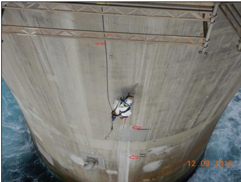
Figure 4-3: Collection of concrete cores from the outside of the seawater shaft. [Equinor, 2018]
