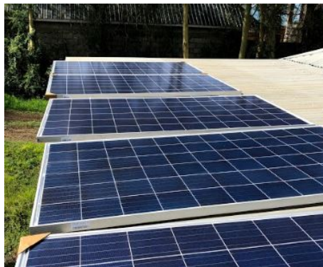
Figure 18: PV panels placed on the roof of the workshop rated 304.1 W and 36.2 V
