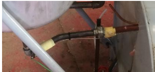
Figure 14: The thermal sensor taped to the pipe for measuring the temperature of the flow out of the cooker
