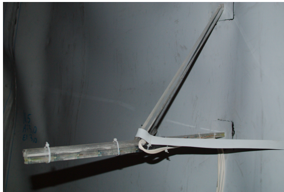
Figure 2.5: Setup of rods before the concrete arch is cast. Extra support was installed in the horizontal and vertical direction to prevent rotation or other movements of the rod under the construction of the arch (Torgeir Jensen, SINTEF).
