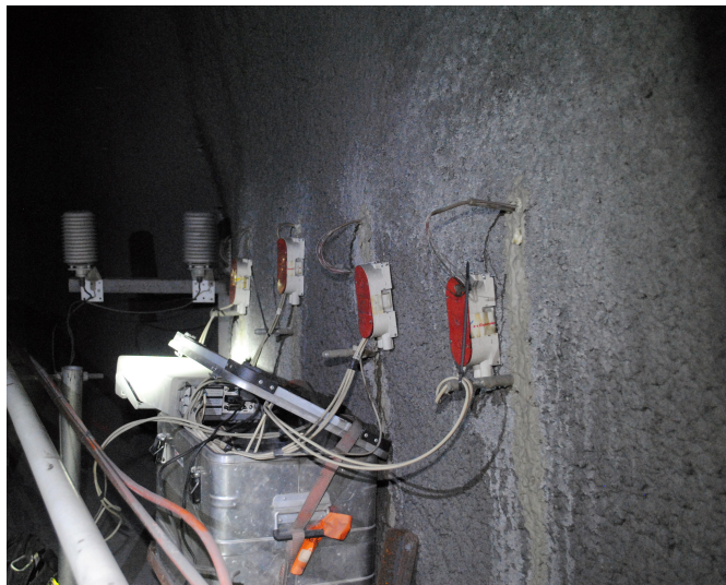
Figure 2.17: Picture from the Gevingås Tunnel showing the measuring installation at the tunnel wall (Date: 01.02.19)
