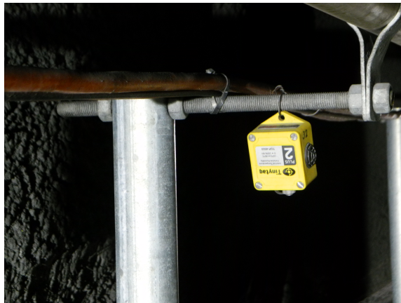
Figure 2.18: Tinytag sensor installed in the Gevingås Tunnel (Karl Gunnar Holter).
