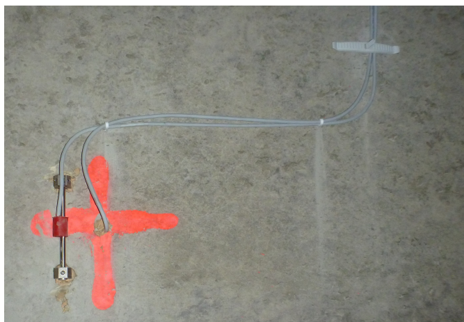
Figure 2.10: Picture of surface sensors in the Ulvin Tunnel, shows the hole leading to the concrete measurements and the surface sensor (Atle Gerhardsen, Cactus Geo).
