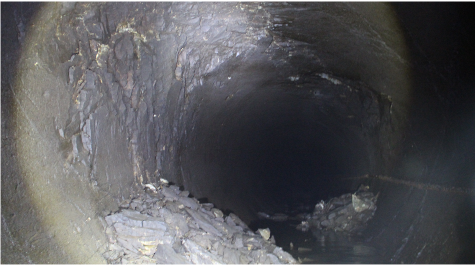
Figure 6.19: Weakness zone in the headrace tunnel 650 m downstream of the Sverjesjøen shaft.
