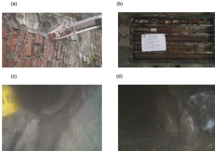
Fig. 12 – Drilling and boroscopy procedure for each investigated location. (a) Core drilling. (b) Cored samples. (c) Visual inspection inside the core. (d) Visual inspection at the core end.
