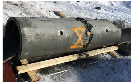
(b) Cracking on pipe with visible fragmentation in the centre.
