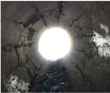
(a) Inside pipe cracking
