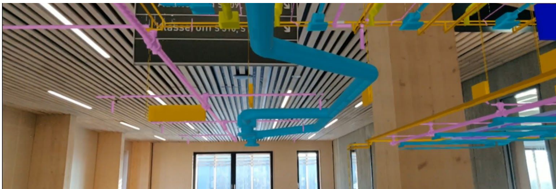
Figure 17: The NTNU S-Building's HVAC and Electrical Layer in AR in the Application
