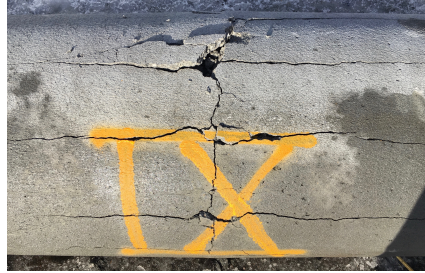
(b) Reinforced BASAL Falsrør ig subjected to 400 g C 4 . Exterior cracks visible in longitudinal and circumferential direction.
