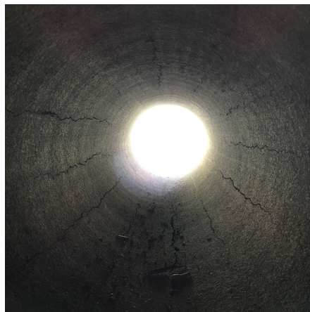
(c) Reinforced BASAL Falsrør ig subjected to 300 g C 4 . Interior cracks visible in longitudinal direction.
