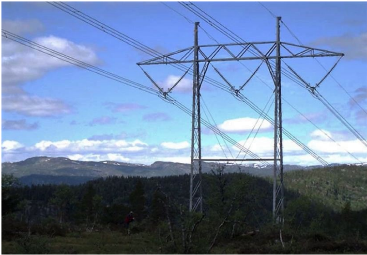
Figure 3.5: Configuration of three conductors and two ground wires. The left line with duplex conductors and the right line with triplex conductors (Statnett).
