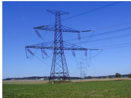
(b) Angle-strain lattice steel tower.
