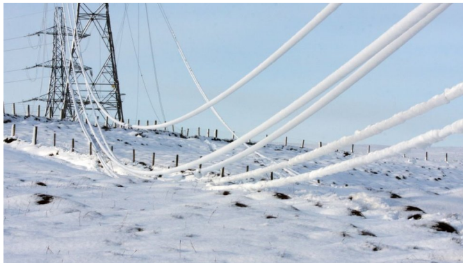
Figure 4.1: Ice on transmission line
