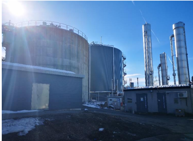
Figure 2: Mjøsanlegget's old and new digester (front and back respectively) and gas washers to the right.
