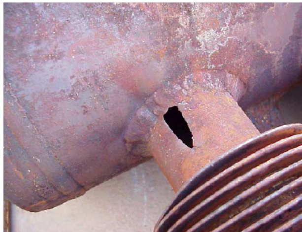
Figure 2.4: Flow assisted corrosion causing economizer tube failure. Source: Intertek AIM, The Increased Cost of Cycling Operations at Combined Cycle Power Plants
