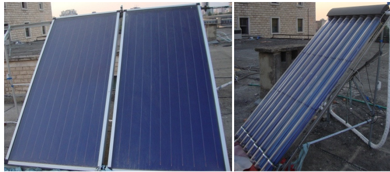
Figure 1. View of the utilized solar collectors
