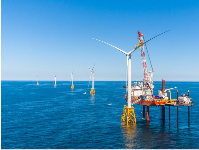
Figure 1: Illustration of system components for offshore single blade installation (DEEP-WATER WIND, 2019) (Note: the jack-up vessel graphically represents the crane vessel in the system components. A floating crane vessel is used in the case study. )
