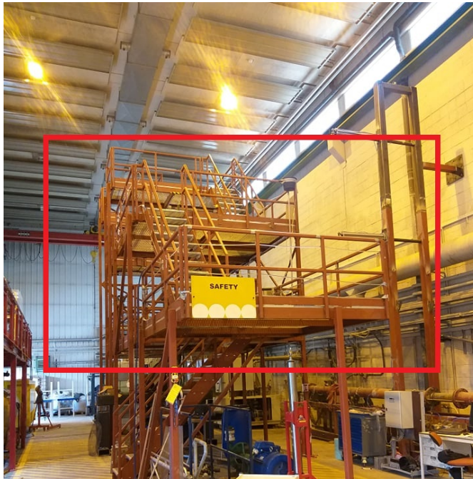
Figure 5.5: Shows the structure the tube is fixed to.
