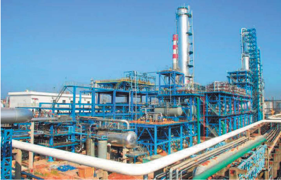
Fig. 3. External view of atmospheric and vacuum distillation unit
