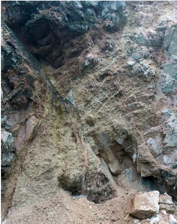
Fig. 15 Road cut just outside Drammen. This weakness zone crosses the Kleivene tunnel on highway E18.
