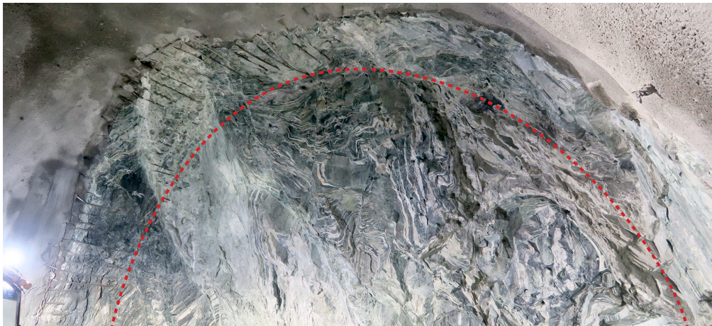
Fig. 4 The weakness zone where the material for sample series 2 was collected, E39 Svagatjørn – Rådal, located in Bergen, Norway. The red dashed line is the approximate location of the transition between the walls/roof and tunnel face. Exposed spiling bolts can be seen in the left wall and in the roof
