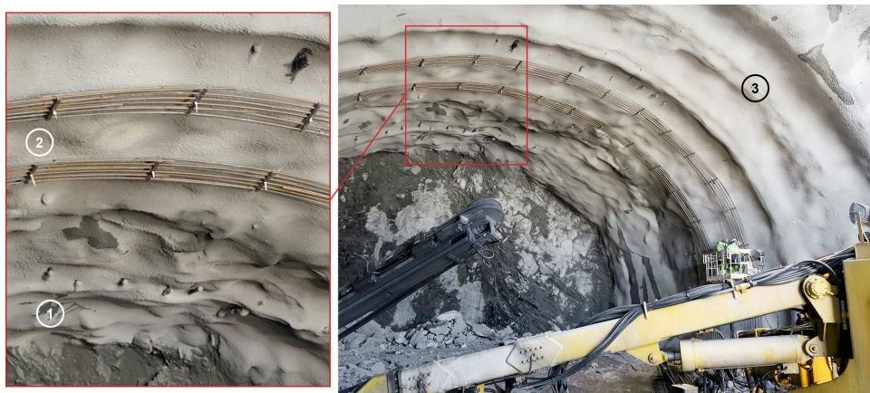
Fig. 1 Mounting of rebars for two RRS for permanent support (2). Further toward the face, two (1) blast rounds are temporarily supported with spiling bolts held in place by steel straps and radial rock bolts. The finished RRS is shown to the right (3).
