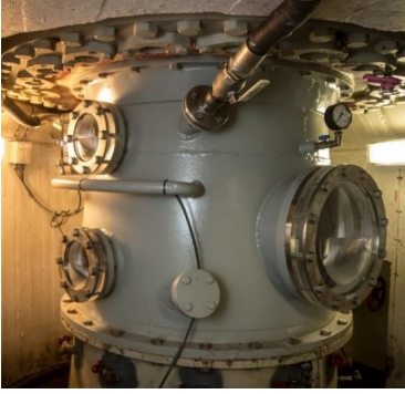
Figure 3. Draft tube at Svorka power plant with acrylic glass windows installed.
