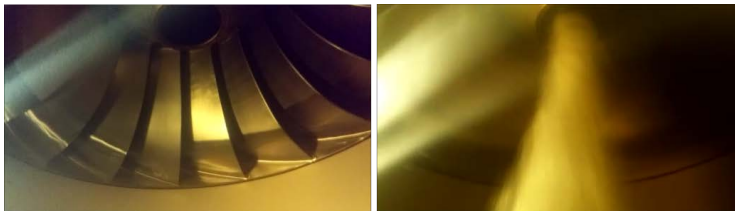
Figure 3. Vision of the runner from the manhole with the machine stopped (a) and with the machine operating at 19 MW (b).
