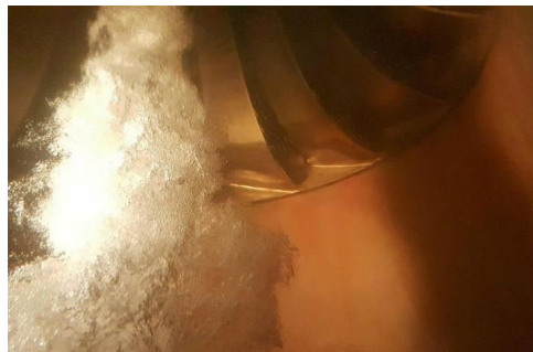
Figure 5. View of the runner and output flow through the man-hole window during operation (photograph by Statkraft).
