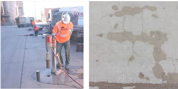
Fig. 14. Coring at the Picton site (left) and surface cracking on the HA pavement section (15 years) (courtesy of R.D. Hooton).
