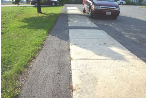
Fig. 11. Sidewalk sections dedicated to ACR testing in Kingston (Canada) (photo by Fournier, 2005).
