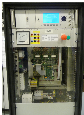
Figure 27: One of the VSC converters.
