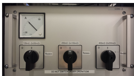
Figure 26: Variable resistor cabinet to emulate DC cable.
