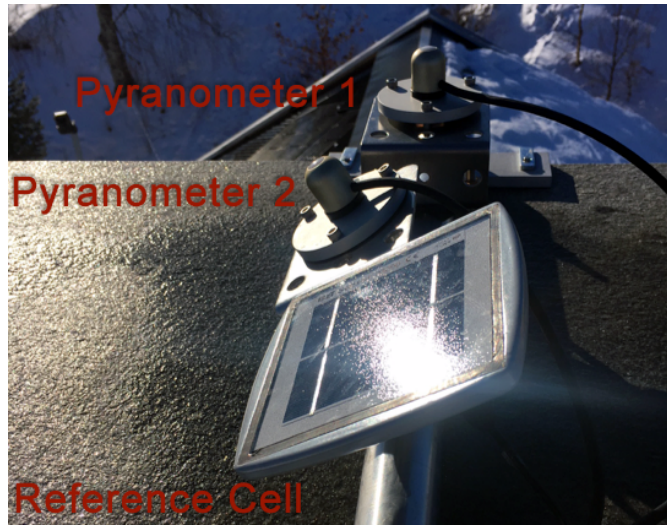
Figure 4.3: Pyranometer 1, 2, and reference cell installed at test site.
