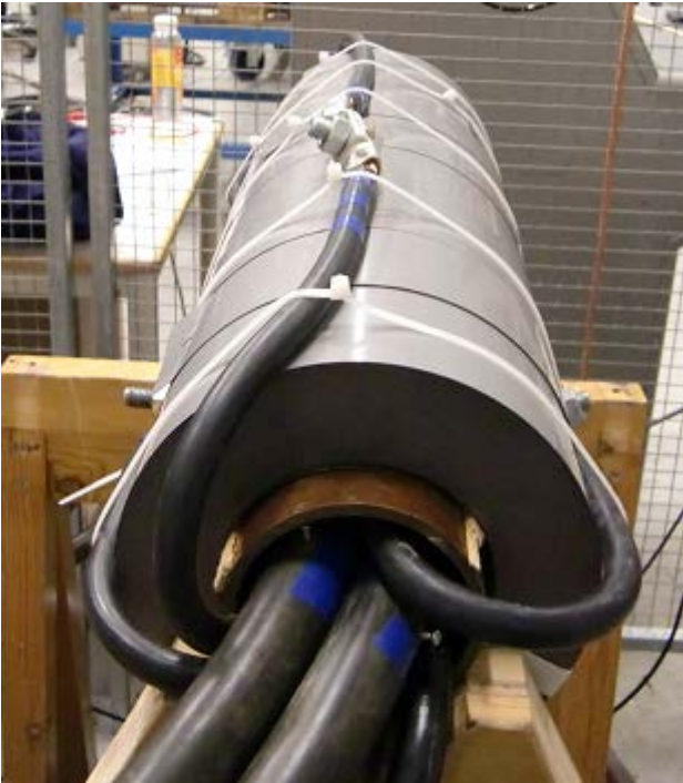
Figure 13-3: Large transformer; side view of the short-circuit assembly
