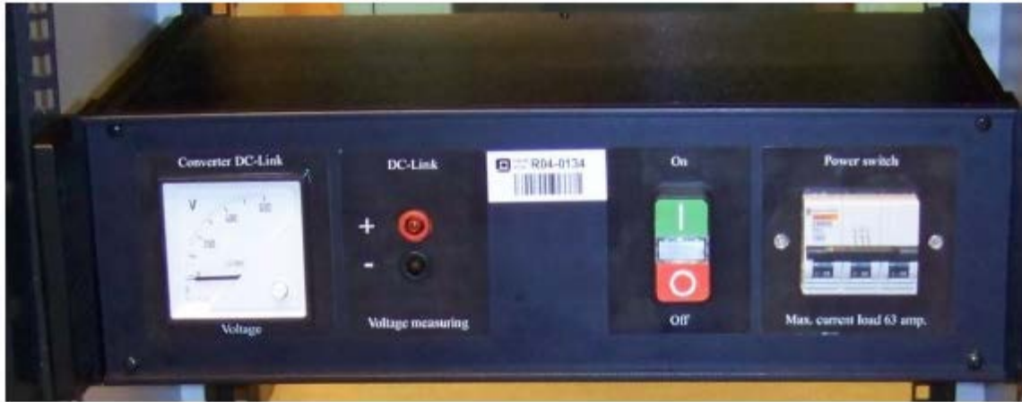
Figure 5-5 Rectifier used in the lab.
