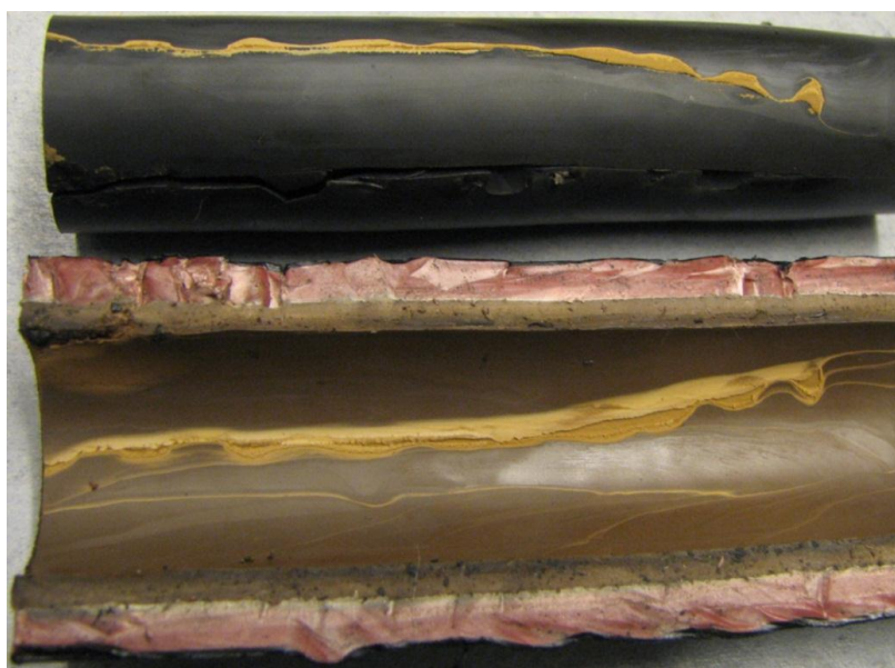
Figure 46. Stress control tube pulled apart from the joint body leaving marks in the joint body material.
