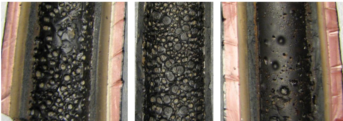
Figure 47. Pits and cavities in mastic between joint ferrule and stress-control tube. Comparison between joints # 1, 2 and 3 (from left to right). A clear difference in the amount of pits in the mastic can be seen between the different joints.
