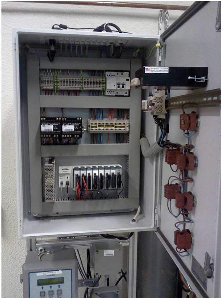
Figure 2.2-1 Electrical connections and instrumentation locker
