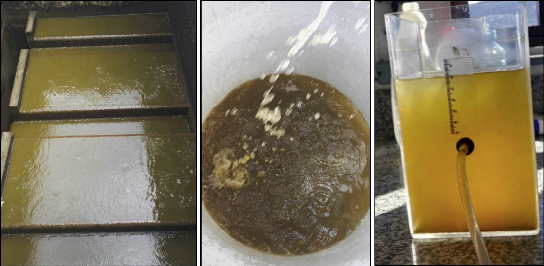
Figure 38: Pictures showing backwashing of filters, and collected backwash water
