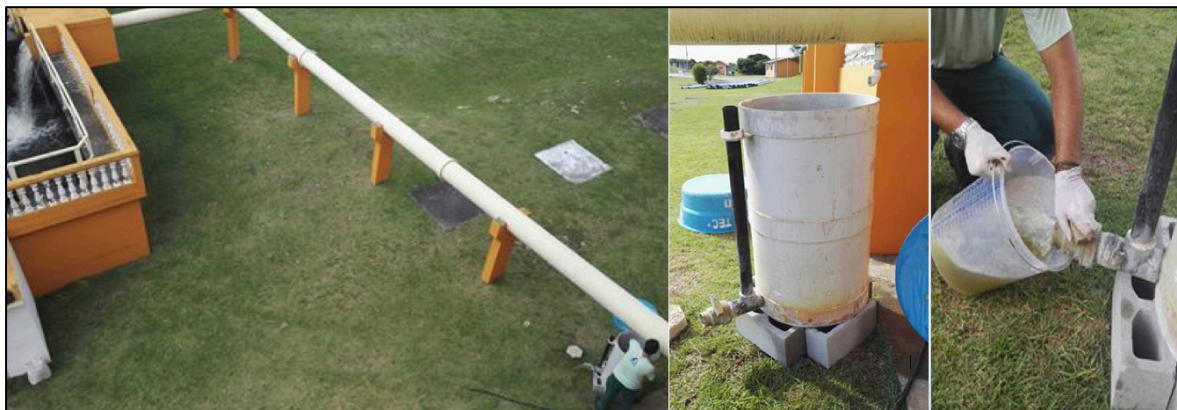
Figure 22: Collection of backwash water at Lake Peri WTP
