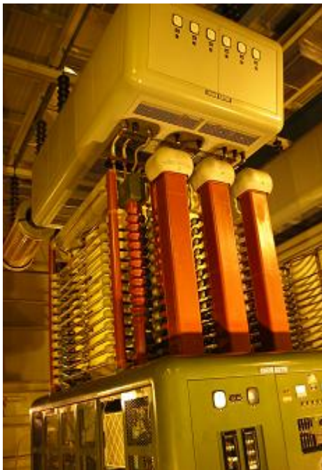
Figure 27 English Electric mercury arc valves at the Manitoba Hydro Radisson Converter Station
