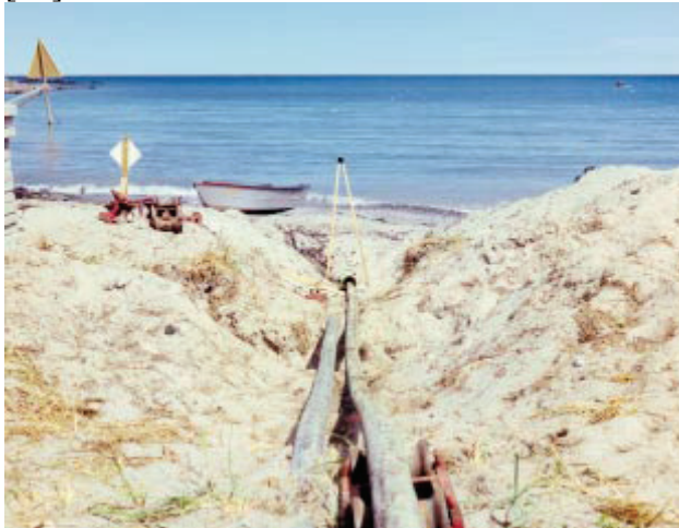
Figure 6 First submarine XLPE cable. (Source: ABB)
