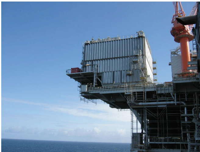
Figure 17: HVDC Light converter station at the Troll A platform. (Source: ABB)
