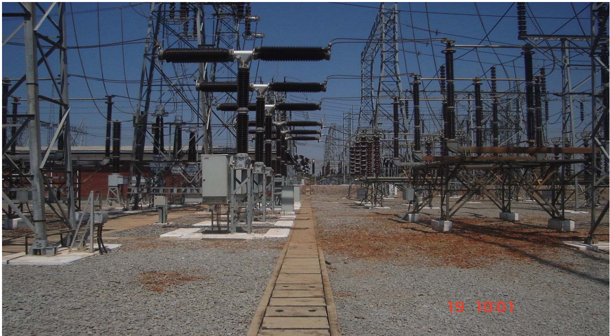
Fig 5 330kV SF6 circuit breakers type FXT15 at Leopards Hill substation
