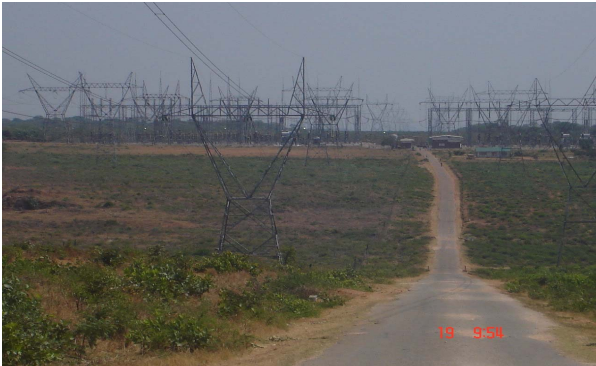
Fig 3 Kariba and Kafue gorge 330kV lines at Leopards Hill substation
