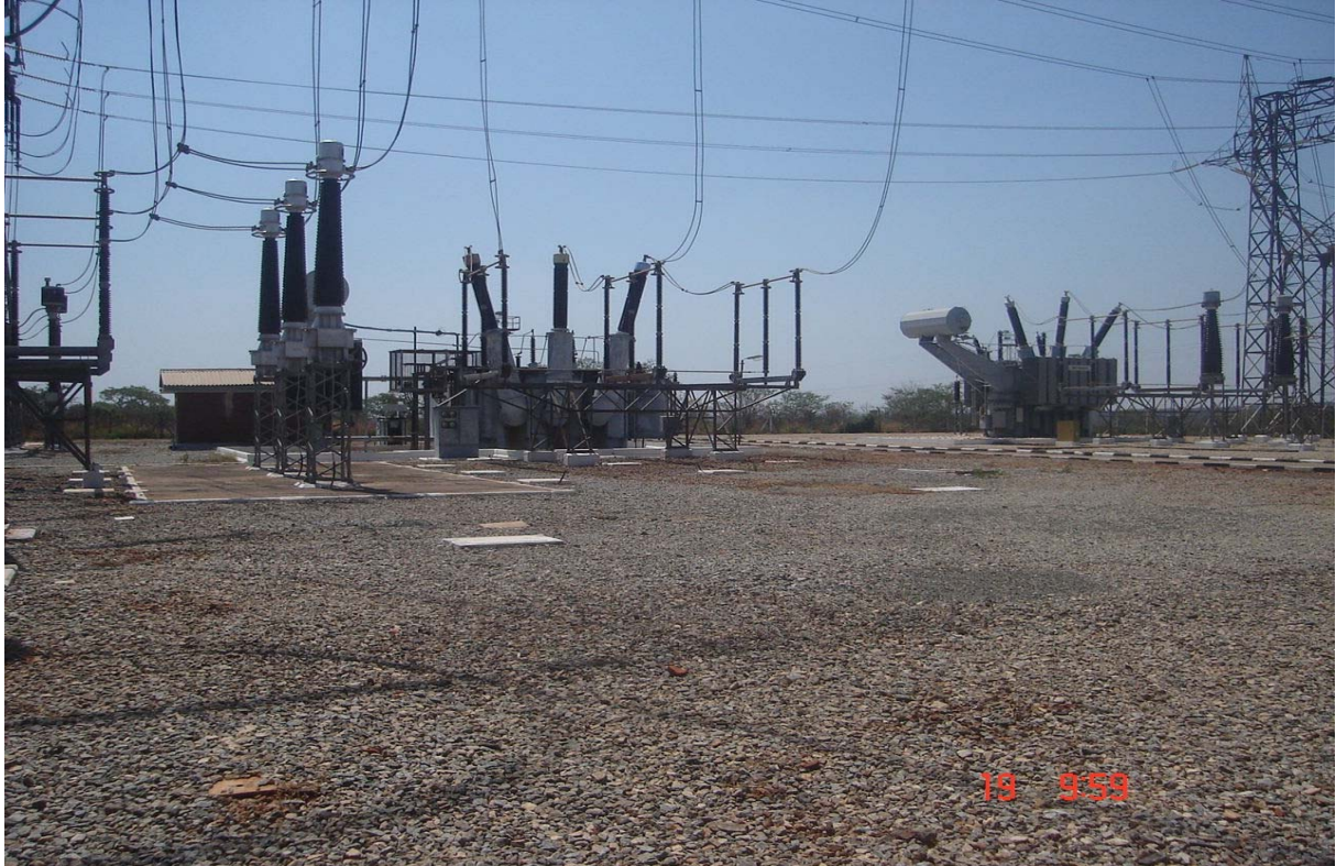
Fig 4 330/132kV transformers at Leopards Hill substation
