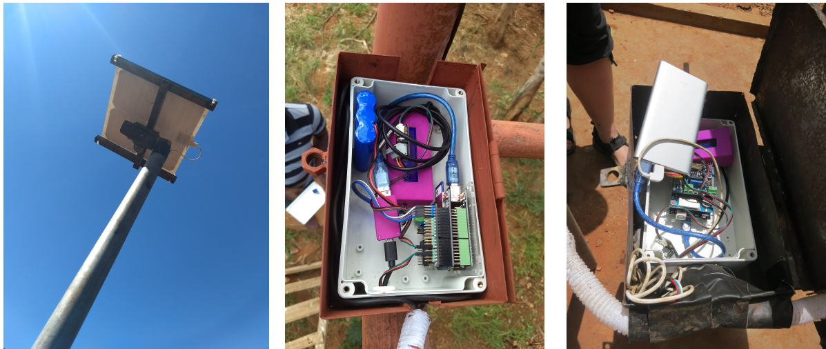
Figure 5-4: 1: Solar panel providing electricity to the system. 2 & 3: the whole system inside a protective metal box.
