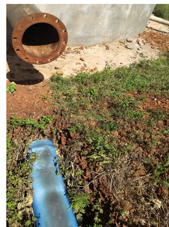
Figure 7-6: PVC pipe lying unprotected after several years of project delay.
