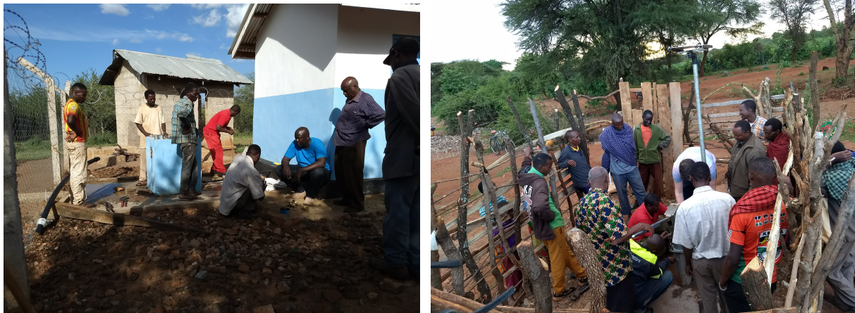
Figure 7-5: Trained technicians and villagers installing sensor in 1: Munguli and 2: Gidarudagaw.
