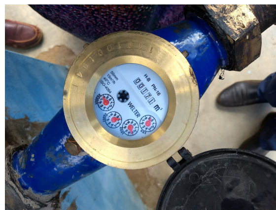
Figure 4-4: Conventional water meter used in Munguli.
