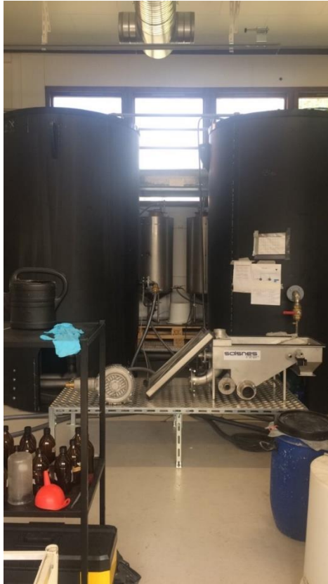
Figure 28 - The two holding tanks where wastewater is pumped in. In the front the Salsnes filter which is in the process of being installed is visible.
