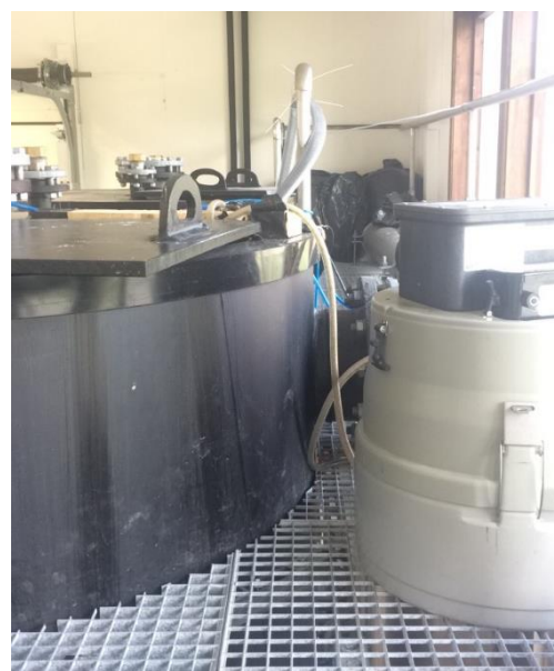
Figure 32 - The automatic composite sampler for influent water placed next to the top of the holding tank
