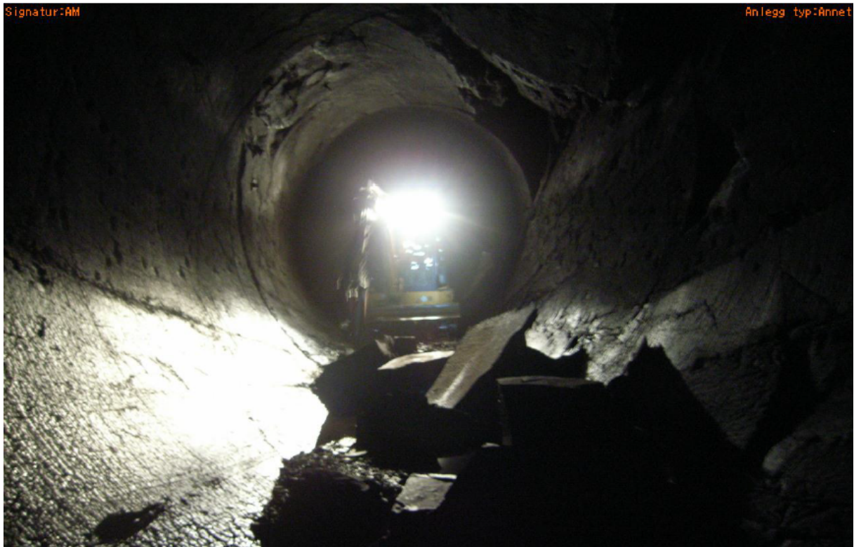
Figure 7.16: Large block fall on Ch. 10 400 in 2015. The large volumes may have been caused by fracturing in the roof that developed and intersected a joint or seam in the tunnel wall (Landløpet, 2015).
