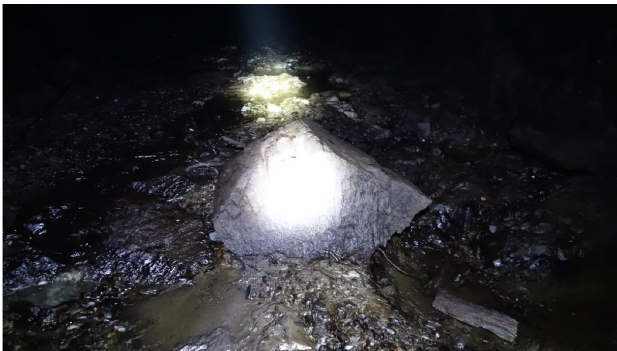
Figure 7.15: Block fall from tunnel roof, downstream the pressure shaft (Landløpet, 2015).
