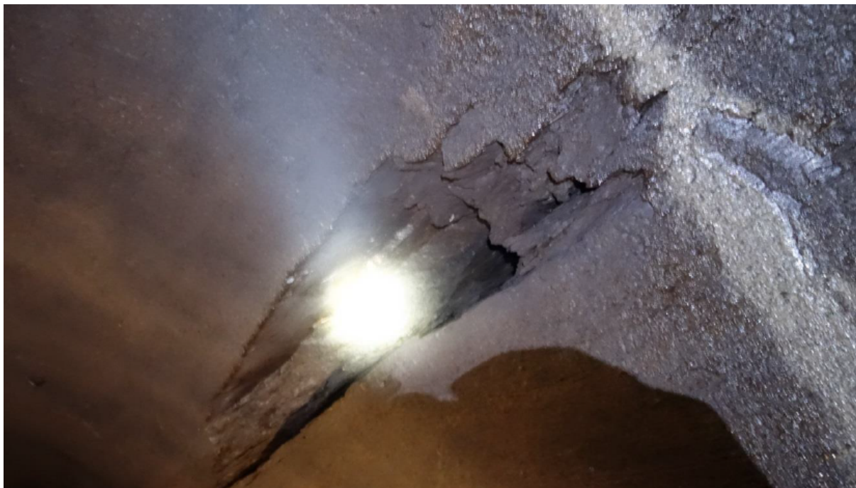
Figure 11.1: Washed-out seam detected during tunnel inspection in 2015. The seam is following the schistosity plane, dipping into the tunnel (Landløpet, 2015).
