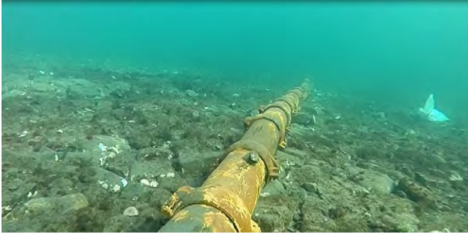
Figure 5: Cast iron from Bell island submarine cable [64].
