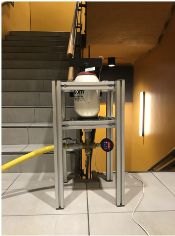
(a) Accumulator in stairwell
