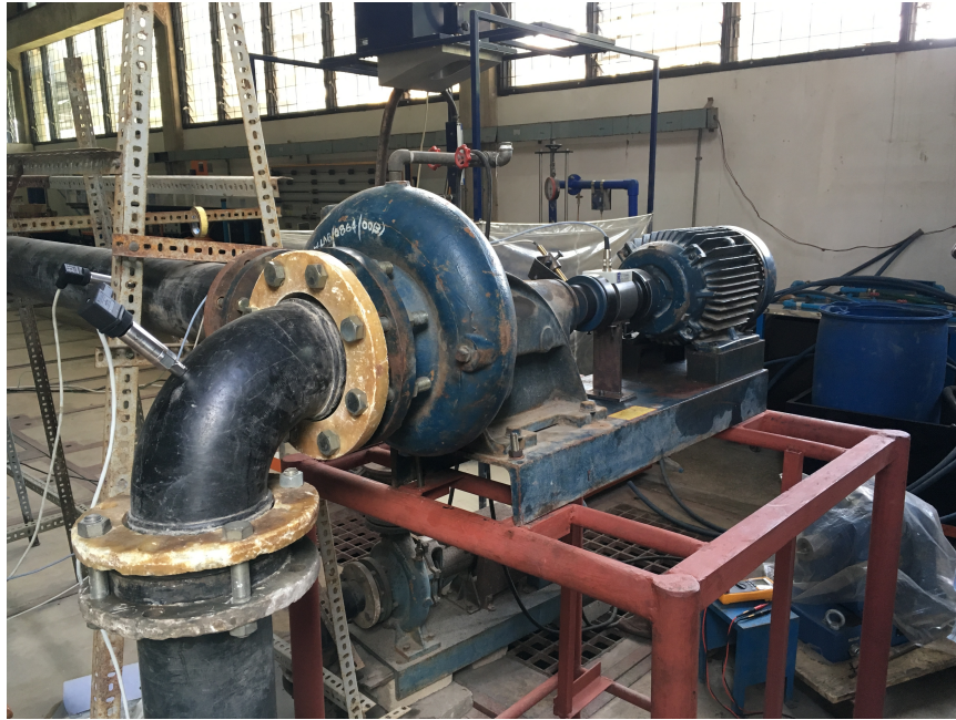
Figure 3.2: PAT test rig at UDSM: Water enters the PAT from the left in the picture, and exits in the foreground. To the right the shaft goes from the PAT to the generator, with a torque transducer in between.
