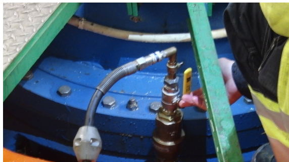
Figure 3.10: Air hose and valve mounted in place of the check valve
