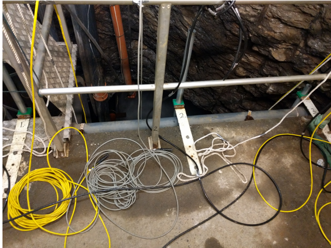
Figure 4.4: Three measuring pipes in outlet
