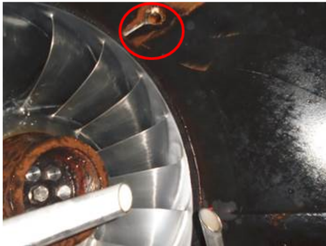
Figure J.2: The broken air injection tube (Statkraft International, 2017)
