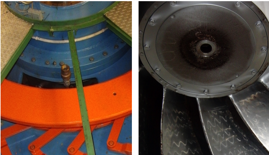
Figure 3.8: Check valve at the turbine cover (left), air vent in the runner centre (right).
