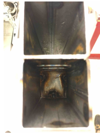
(b) Leaks formed around the separation plate in the outlet chamber.
