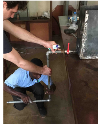
(c) The piping system, with a bullet valve, from the heat storage to the cooking application.
