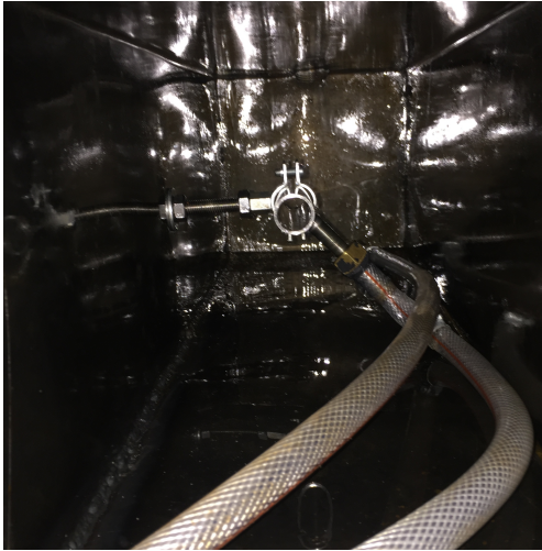
Figure 4.8: Fill valve inside the cold section
