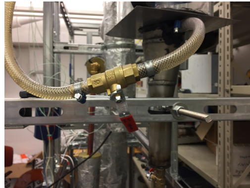
Figure 3.4: Inlet control valve
