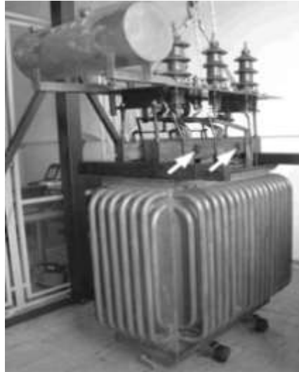
Figure 24. Transformer presenting a first degree mechanical defect of the active part (Borucki, 2012)
