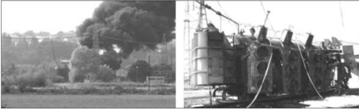
Figure 20. Catastrophic transformer failure (Borucki, 2012)
