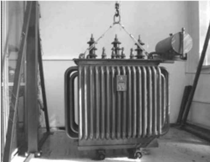
Figure 22. Power transformer under study (Borucki, 2012)
