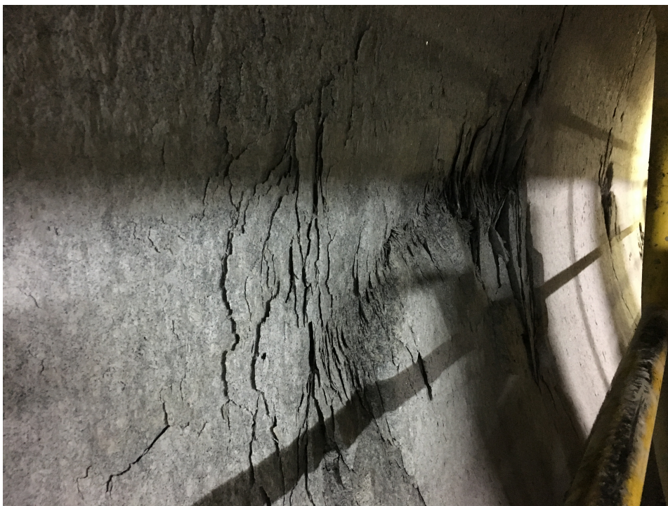
Figure 44: Spalling of rock mass at chainage 8170 (Photo: O. Hobbelstad)
