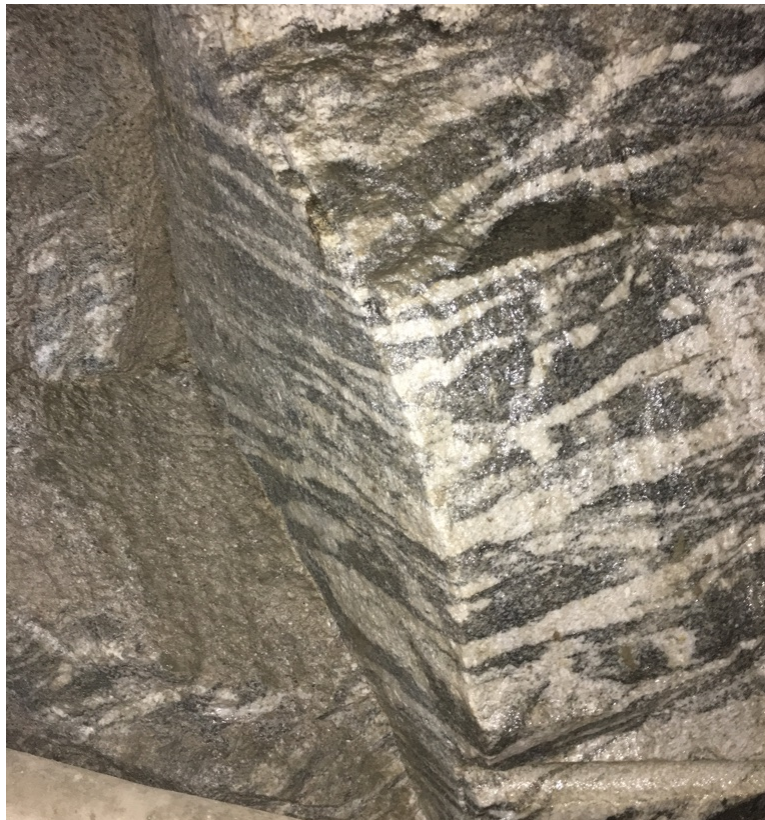
Figure 24: The jointing of the rock mass in the portal tunnel (Photo: O. Hobbelstad)
