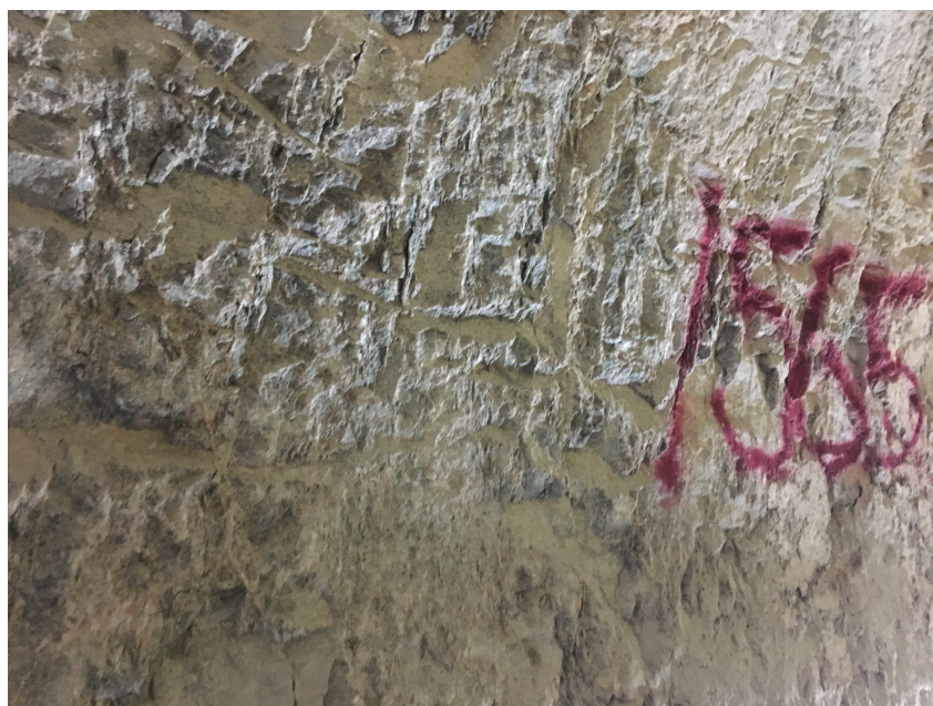
Figure 41: Very uneven surface, approx. 2,5 x 2 meters (Photo: O. Hobbelstad)
