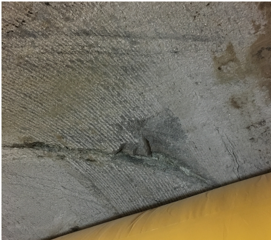
Figure 45: Fallout of wedge between steep joint intersected by a fracture (Photo: O. Hobbelstad)
