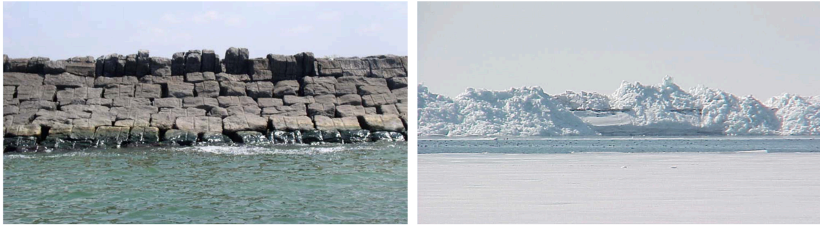
Figure 2-6 Breakwater in Buffalo, NY, USA. Left) Summer conditions showing the smooth armor placement. Right) Winter conditions showing both ride-up and pile-up (Michael Mohr as found in Sodhi 2014 [19]).
