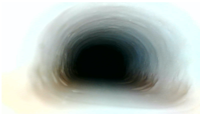
Figure 7.24: Picture taken 15cm inside copper pipe, outlet side
