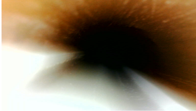
Figure 4.6: Picture 15cm inside copper pipe, inlet side
