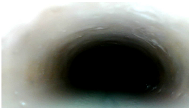
Figure 7.12: Picture taken 15cm inside copper pipe, outlet side
