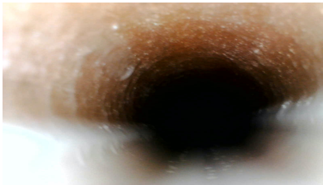
Figure 7.2: Picture taken 15cm inside copper pipe, inlet side
