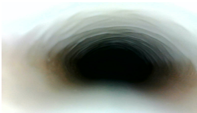
Figure 7.36: Picture taken 15cm inside copper pipe, outlet side
