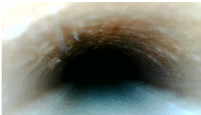
Figure 7.30: Picture taken 15cm inside copper pipe, outlet side
