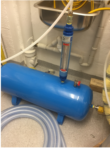
(a) Pressure Tank and Techfluid Flow Meter
