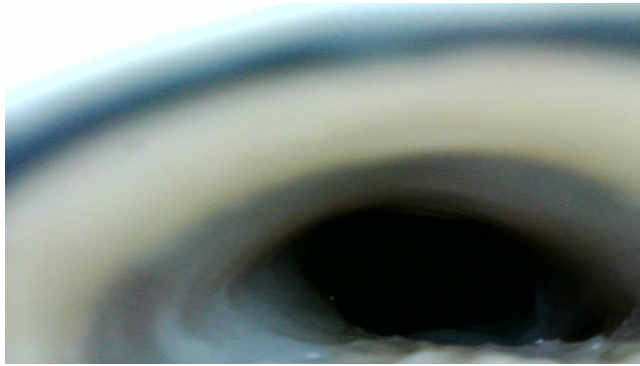
Figure 7.21: Picture taken 15cm inside copper pipe, outlet side
