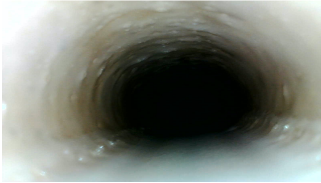
Figure 7.5: Picture taken 15cm inside copper pipe, inlet side
