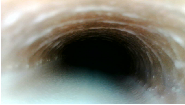
Figure 7.3: Picture taken 15cm inside copper pipe, outlet side
