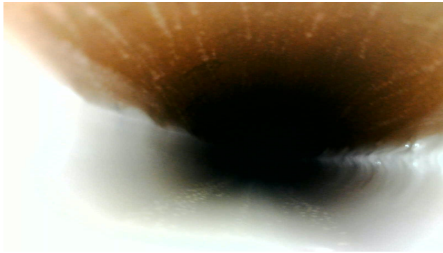
Figure 7.35: Picture taken 15 cm inside copper pipe, inlet side
