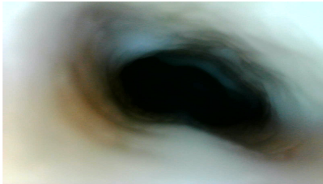
Figure 7.15: Picture taken 15cm inside copper pipe, outlet side
