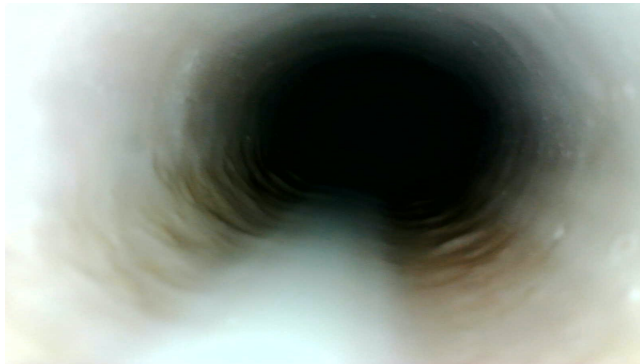
Figure 7.47: Picture taken 15cm inside copper pipe, inlet side
