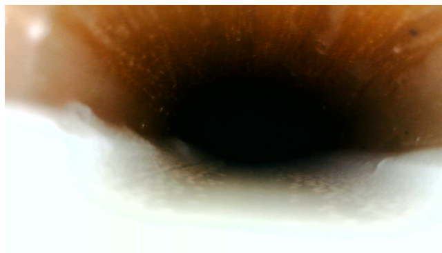
Figure 7.20: Picture taken 15cm inside copper pipe, inlet side
