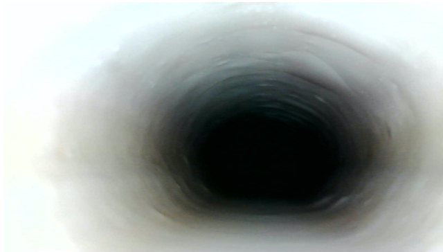
Figure 7.17: Picture taken 15cm inside copper pipe, inlet side
