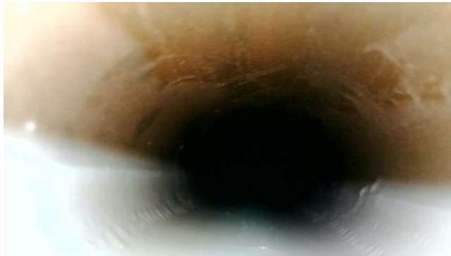
Figure 7.41: Picture taken 15cm inside copper pipe, inlet side
