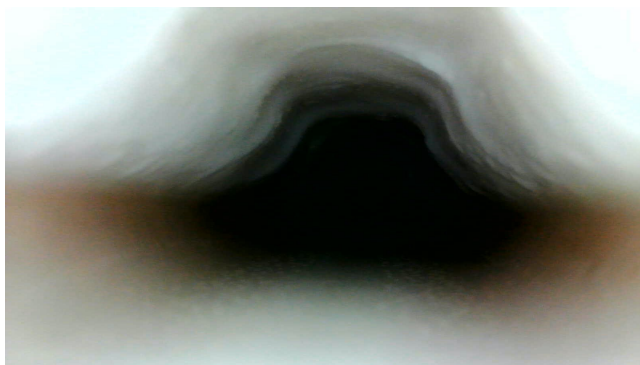
Figure 7.42: Picture taken 15cm inside copper pipe, outlet side
