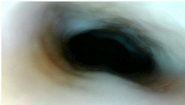
Figure 4.13: Picture taken 15cm inside copper pipe, outlet side under wavy stratified flow
