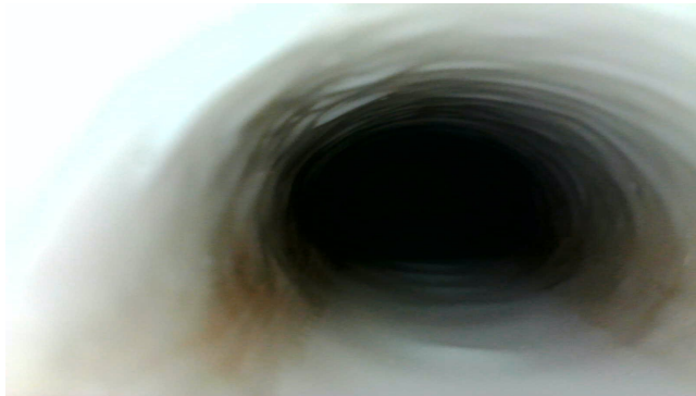
Figure 7.45: Picture taken 15cm inside copper pipe, outlet side
