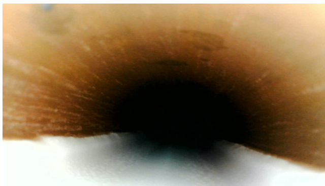
Figure 7.26: Picture taken 15cm inside copper pipe, inlet side
