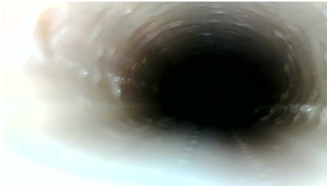
Figure 7.6: Picture taken 15cm inside copper pipe, outlet side
