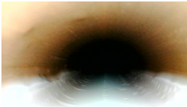
Figure 7.38: Picture taken 15cm inside copper pipe, inlet side
