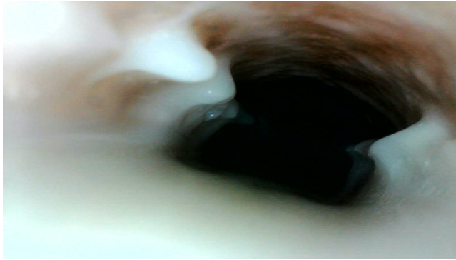
Figure 7.33: Picture taken 15cm inside copper pipe, outlet side
