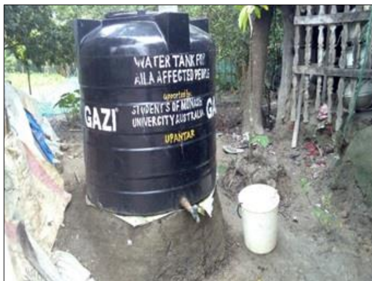
Figure 4:2 Rain water harvesting tank (sample 2)
