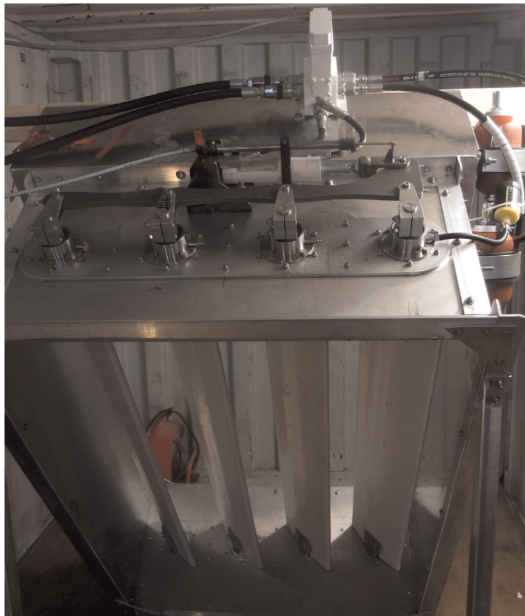
Figure 1.12: Hydraulic actuated vent valve system for the Wave Craft (Courtesy of Umoe Mandal) (Auestad, 2015)
