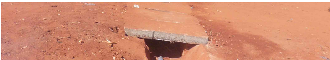
How it was "supposed" to be done: Small bridge that allows free circulation in the drains. Photo: Hilde Refstie
