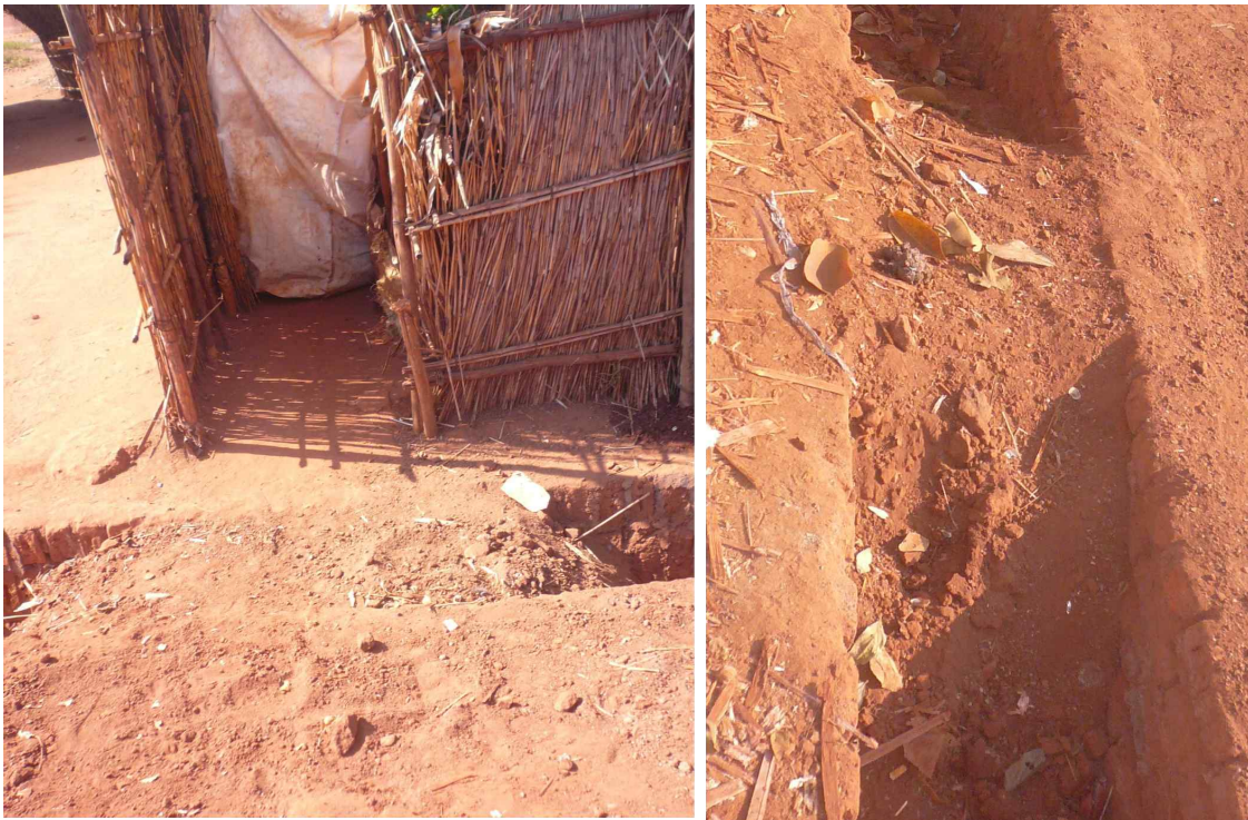
Clogged drains in Chinsapo. Photo: Hilde Refstie
