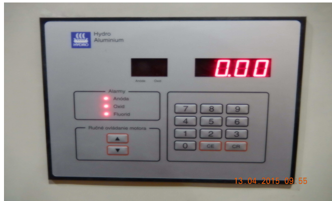
Figure 4.5: Panel on the control cabinet used to run feeder tests
