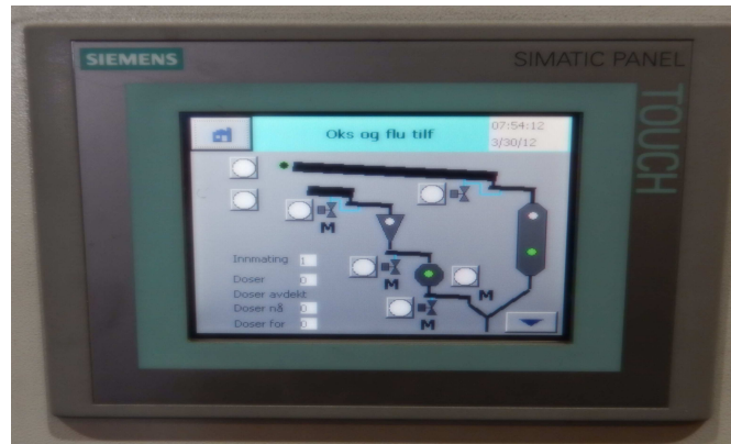
Figure 4.3: Siemens simatic panel used for filling alumina silo supplying the CAS
