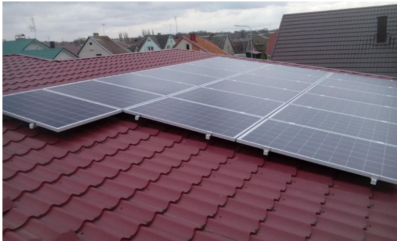
Figure 47. Standard example of 5kW solar module system ( source: “Saulės graža“ archive )
