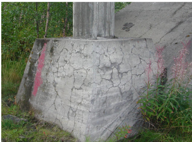
Figure 2. Typical map cracking on the surface of a concrete foundation with alkali-silica reaction (ASR).
