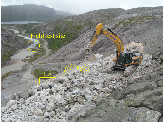
Figure 2.1.: Rehabilitation work at the 129 m high dam Svartevatn. The excavator is setting the placed riprap on the downstream slope of 1:1.5 corresponding to S = 0.67 . The downstream slope and the inclination \beta of the riprap stones are indicated. The field tests site (described in Section 3.2) is marked with a circle (Photo: NTNU).
