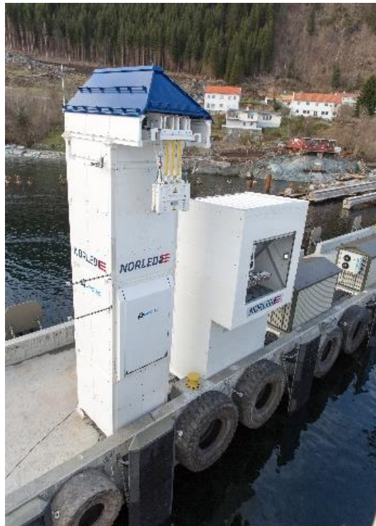
Figure 7: Charging station consisting of plug (left) and pantograph (right) (Siemens AG, 2015)
